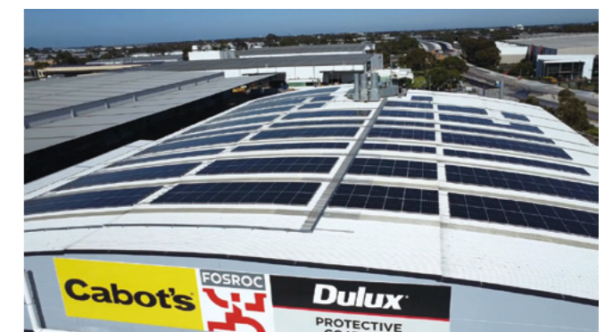
Photo shows solar installation on roof of DuluxGroup Dandenong South factory.
